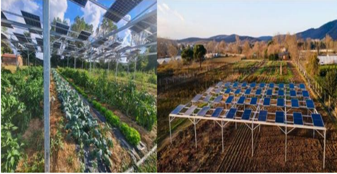
Figure 4. Komşuköy APV System
